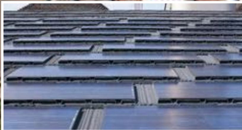
200 Photovoltaic panels on the south-facing roof supplies energy back to the National Grid
